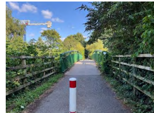
Pedestrian and cycleway with encroaching vegetation.
